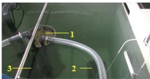
Figure 14: Aerobic tank, with immersed membranes (1), a diffuser for providing air (2) and a recirculation pump (3)
