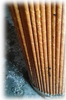
Figure 23: Spare membranes that were clogged because an overdose of Ferric Chloride
