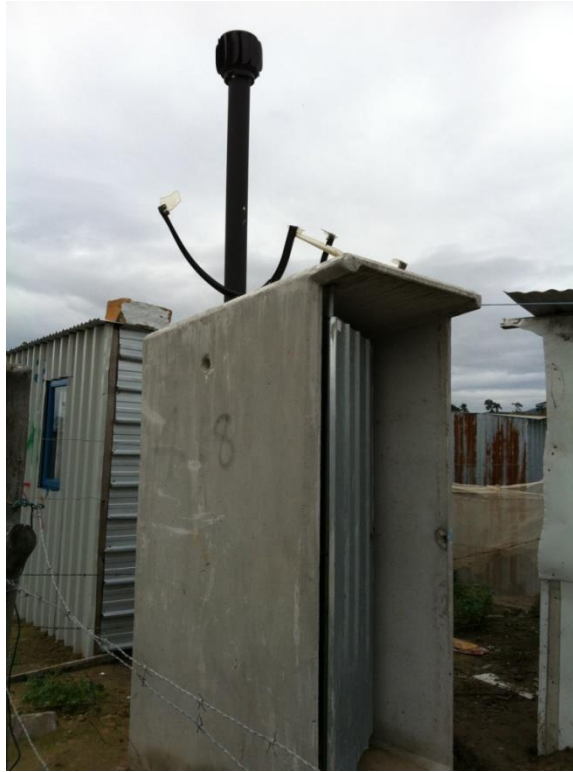
Figure I.3: Afrisan toilet with missing solar panel in Klipheuwel (Pan 18/6/2014)
