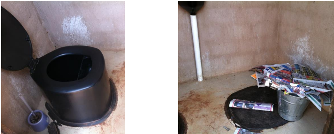
Figure 4.11: UD pedestal, alternate chamber cover, urinal and newspapers for anal cleansing (Pan 20/5/2015)
