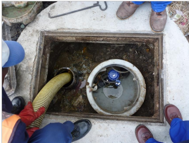
Figure C.7: Overflowing sump in Kosovo requiring the collection chamber to be desludged (Taing, 2010)
