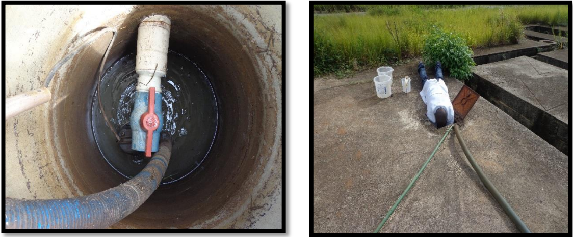
Figure 4.11: Pump and outlet valve for sending the percolate from sludge unit to percolate unit.
