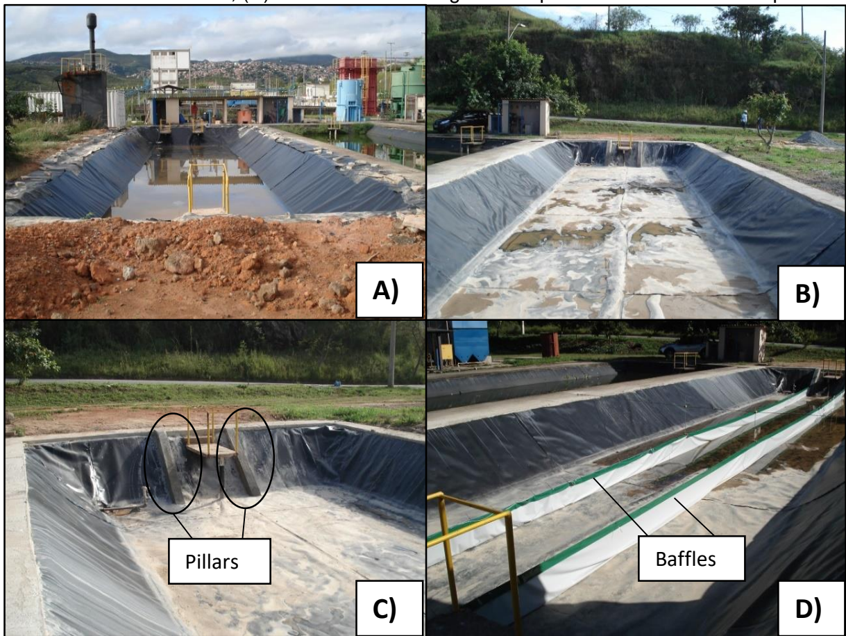
Figure 5.2 - Pond 2 renovation. (A) Desludging and removal of the existing geomembrane canvas (Pond 2); (B) Placement of new geomembrane canvas (Pond 2); (C) Pillars constructed at each end; (D) baffles 90% the length of the pond are anchored to the pillars.
